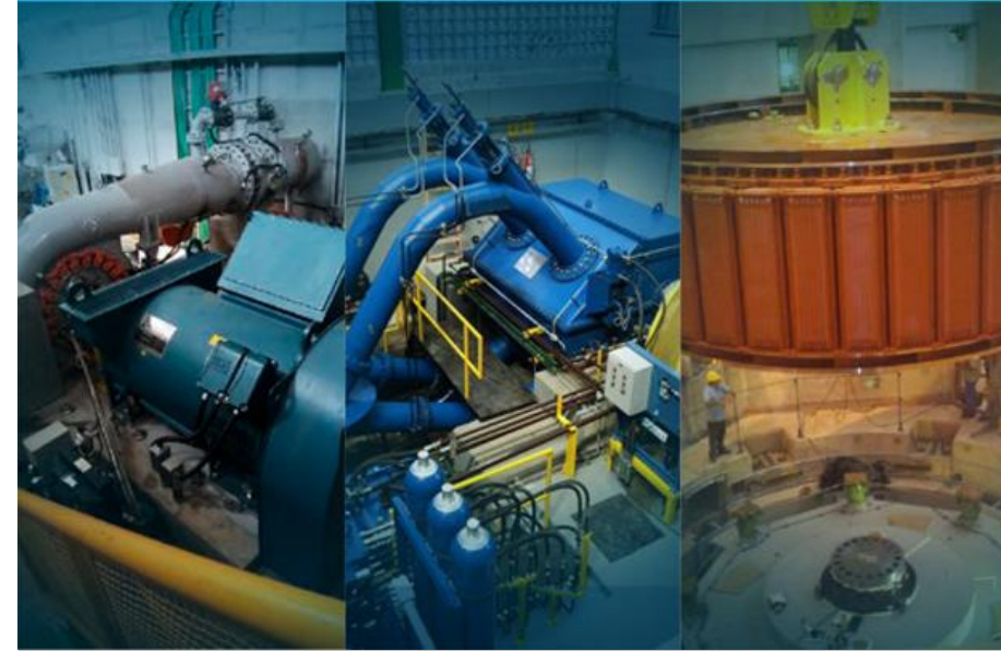
Small Hydro 5 MW
