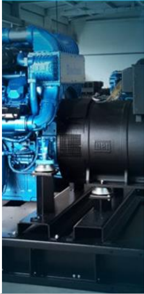
Distributed power generation 25,000 kVA
