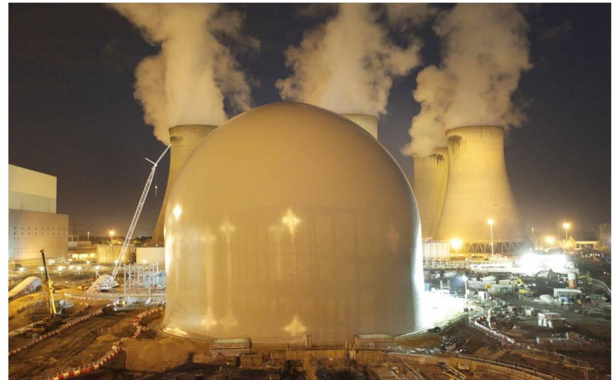
Site storage for up to 350,000 tonnes of biomass pellets in four 63m diameter x 52.25m tall domes at Drax, the largest coal-fired power station in the UK
